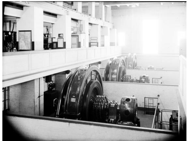
Internal photograph of the substation's ground floor with Siemens Rotary Converters. (Source: Photographic Collection: Railway Negative: Alpha-numeric systems , VPRS 12800, CEE/0439, PROV)
