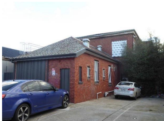
24-26 Derby Road, Former SS Bank. The rear single-storey wing retains intact hipped roof form and slate cladding, whereas it has been removed from the two-storey part.
